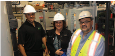
Left to right: Benjamin Moore, Lexus Mechanical; Kim Menard, Centretown Citizens Ottawa Corporation; Stacey Bernier, Corix Utilities
