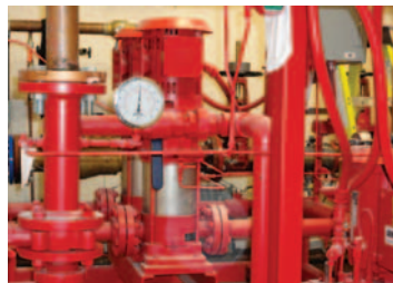
Corix Utilities, central geo exchange plant
